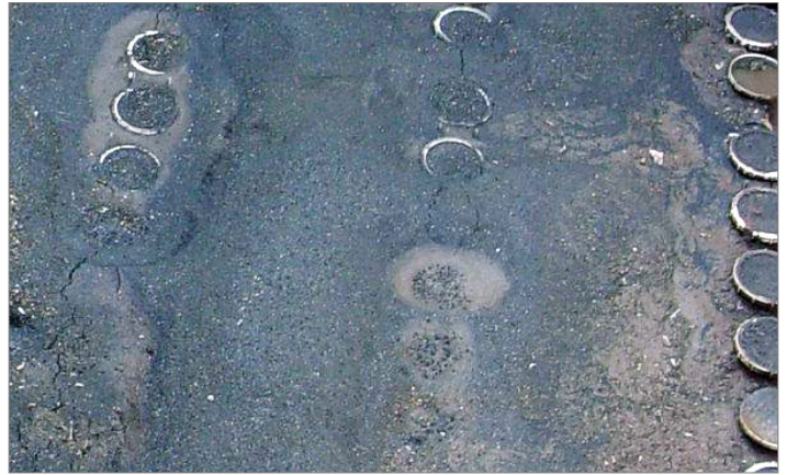
Grit Covered Diffusers Resulting from Ineffective Upstream Grit Removal System
